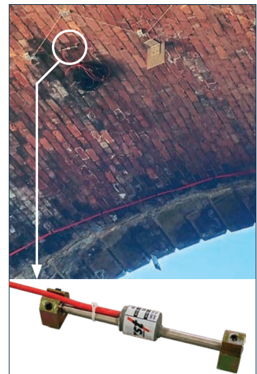
Closeup shown of an RST Vibrating Wire Arc Weldable Strain Gauge. A series of these were installed on the arch of the bridge.
