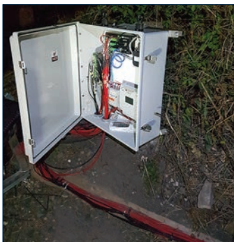
Instrumentation cables (red) leading into data logger.
