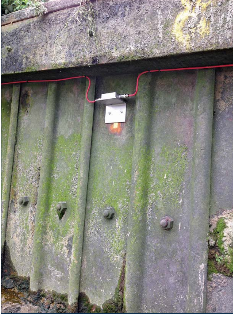
1 of the 3 Digitally Bussed Submersible Tilt Meters along the east retaining wall.
