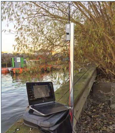
RSTAR Node (DT2485), installed on mast, transmits data wirelessly.
