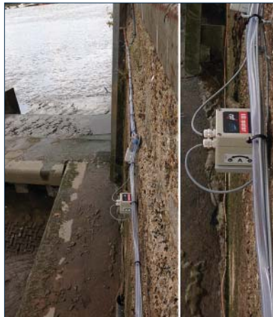
1 of the 8 In-Place Tilt Meters installed along the river walls.
